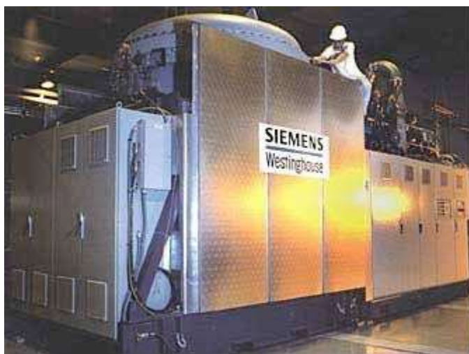
Fig.III.12 Installation Siemens-Westinghouse de Irvine (220kW) (2002)
